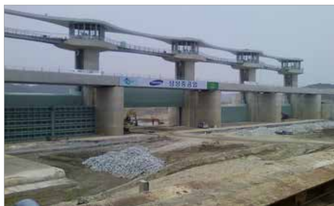
position sensing of flood gates
